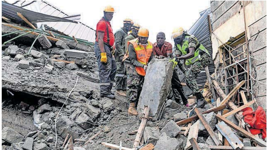
Members of the Disaster Rescue Unit (DRU) from the Kenya Defence Forces (KDF) remove debris of concrete at the scene of a collapsed building, blamed on poor construction materials in Kirigiti, Kiambu County, on September 26. PHOTO | AFP
